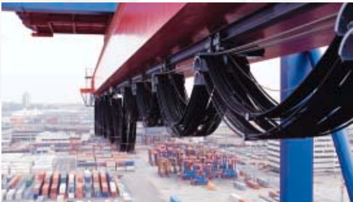
Motorized cable trolley system on a ship-to-shore container crane
