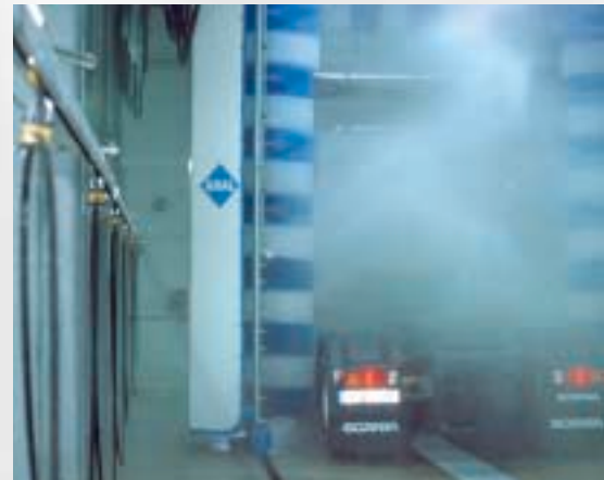
Cable trolley system in a humid environment
