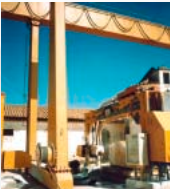
Spring cable reel on a bridge crane
